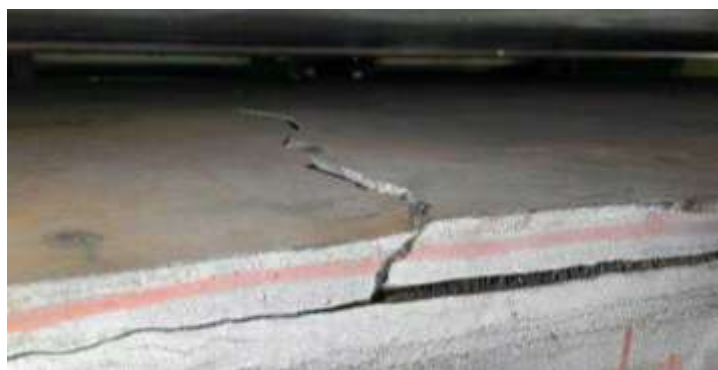
Figure 23 Fracture of the original top beam after 16522 cycles of test
