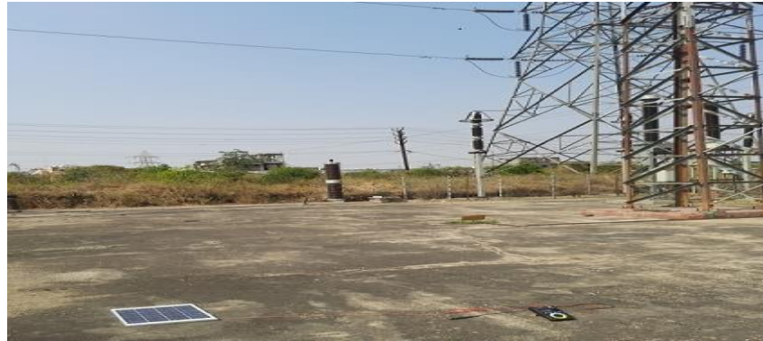
Figure 3. PV module located below the 230kV transmission line.
